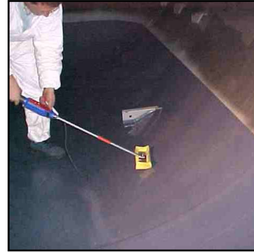
Sponge testing the Belzona ® 1391 to ensure no application defects were present in the coating.
